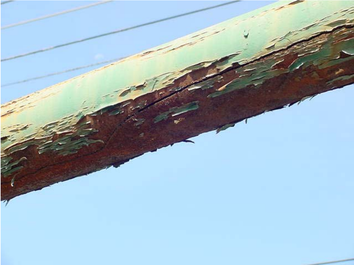
FIGURE 4 Crack in compression arm.
