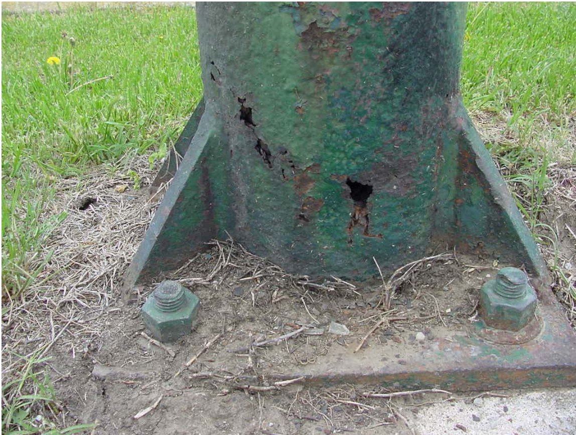
FIGURE 6 Holes above and below rib flanges.
