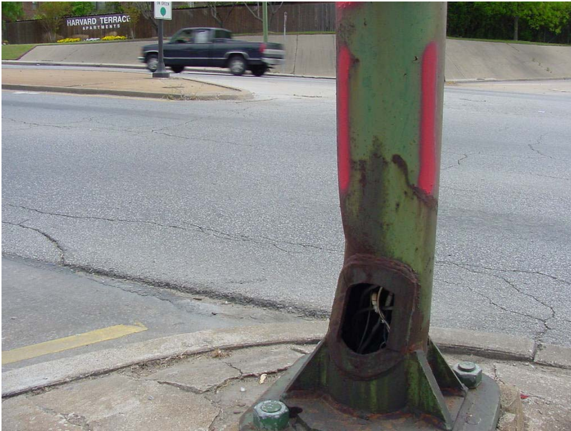
FIGURE 3 Post damaged and in harm's way.
