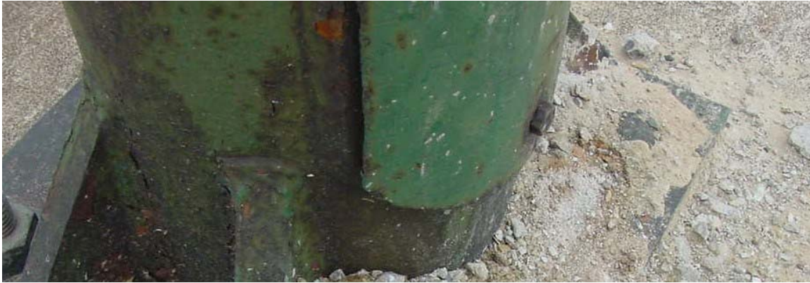
FIGURE 8 Missing anchor bolt.
