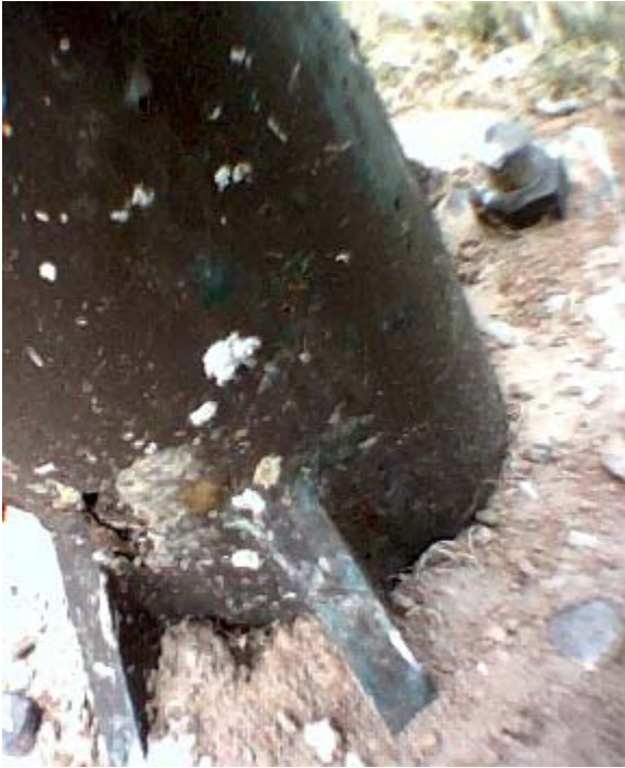
FIGURE 5 Hole in post above rib flanges.
